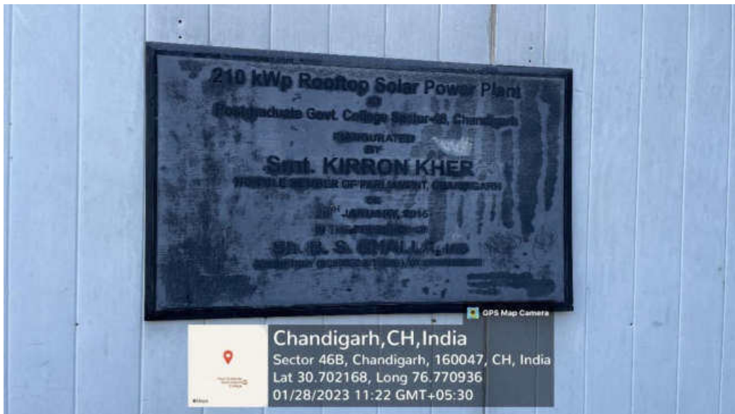
Rooftop Solar Plant
