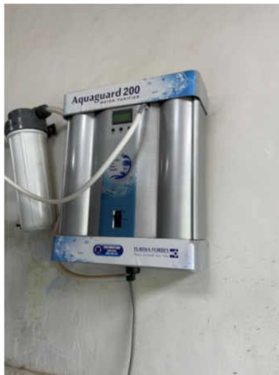
Drinking Water facility in Girls' Common Room
